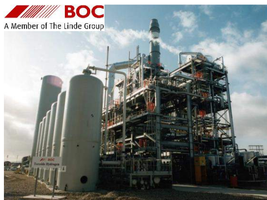
BOC SMR facility, North Tees
